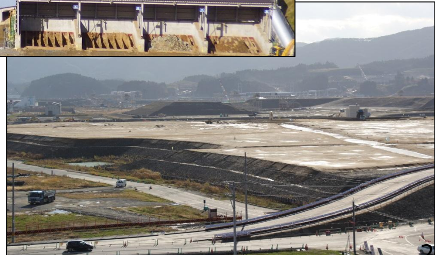
View of Takata district, raising the level of embankments (as of Oct. 2015)
